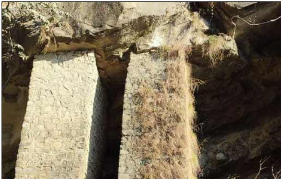
Figure 3: Photograph showing column to support hanging block, a way of mitigation rock fall.
