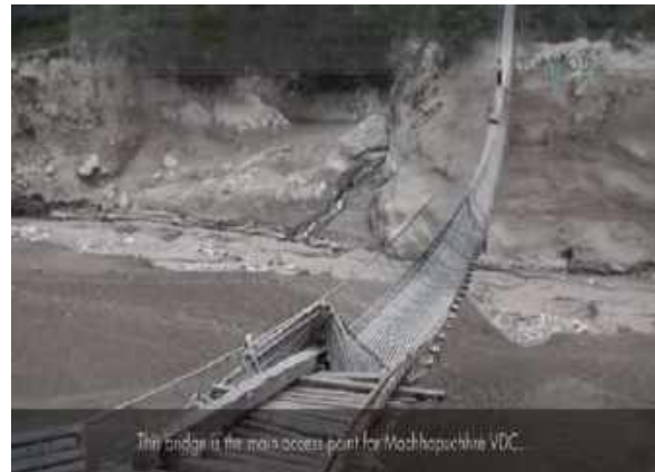
(b) Main bridge damage in Machhapuchhre VDC
